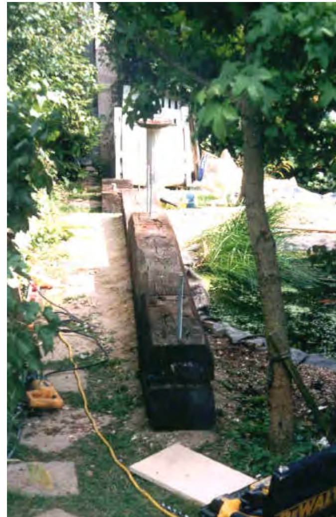
The first couple of sleepers in place. The ballast foundation and steel pins are clearly visible, as is the old pond.
