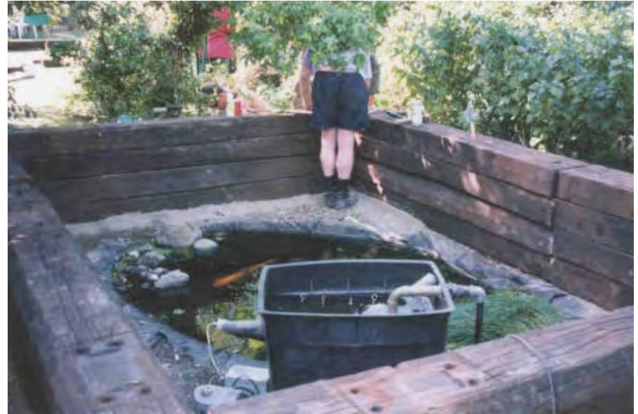
Here the last sleeper has just been laid. In the far corner John considers fitting the first of the cross-bolts. Note a large orange koi looking very out of place.
