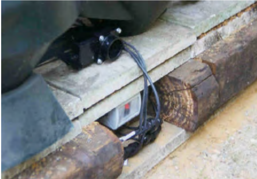
Detail of the electrics. Power is distributed from the waterproof switch box mounted below the filtration unit. All the electrical appliances are removable by disconnecting the waterproof connectors. Note the gate valve on the filter vortex above the switch box, and the base for the filtration system built from spare pieces of sleeper and paving slabs. The switch box was later covered with a spare flap of butyl liner for added weather protection. When draining the filter chambers temporary flexible hosing will be fitted to the gate valves to run the water away from site.
