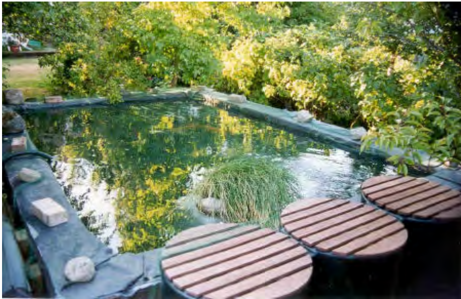
The new pond in evening sunlight a couple of days after completion. Note that the coping is still missing from the walls and net is held in place with bricks. Filter in foreground.
