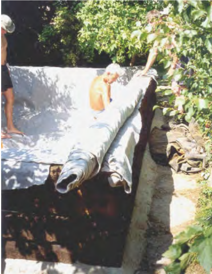
Another view of Keith and Ken fitting the underlay. Notice the old butyl liner on the path at right. Also shown is the concrete skirt which finishes off the dry mix ballast/cement on which the sleepers were laid.
