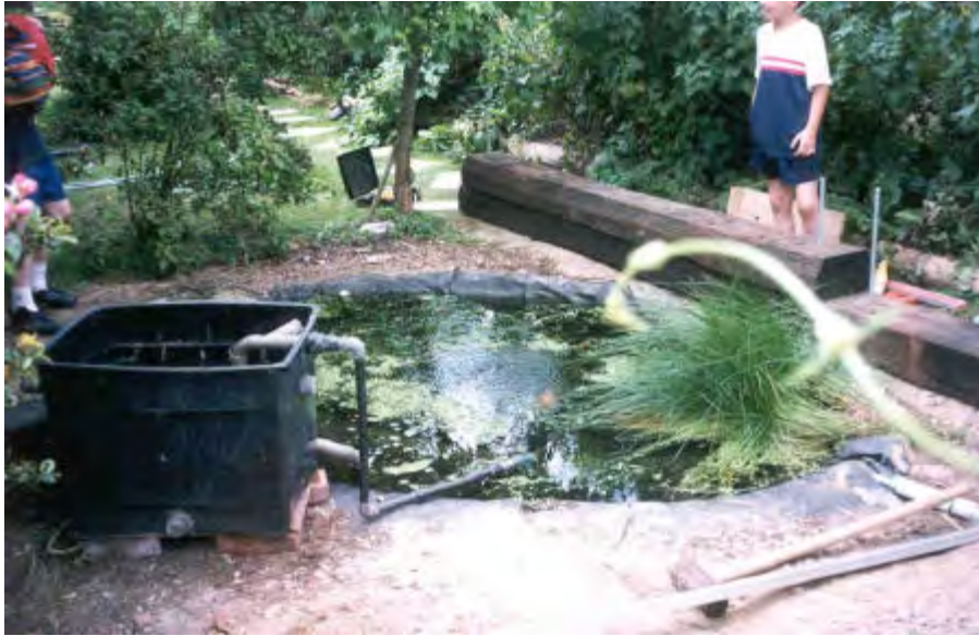
Another view of the first couple of sleepers laid. Despite the young helpers it looked like, and was, a construction site.
