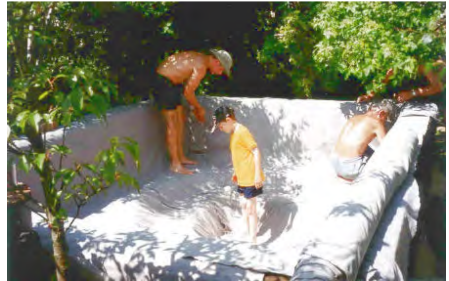
Fitting the underlay: make sure all the joins and folds are neat and secure. [L to R: Keith, Ben, Ken]
