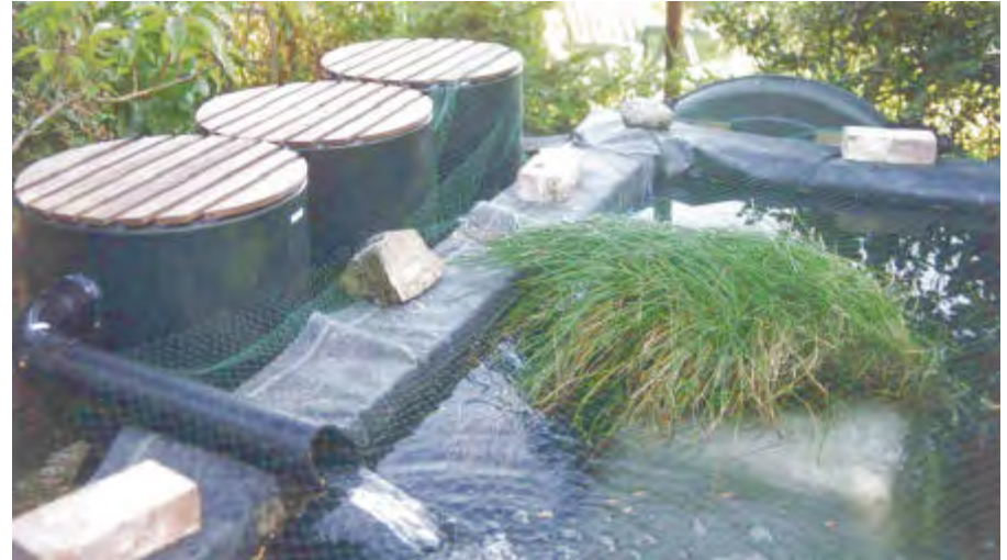
The final construction showing the UV unit (humped shape, back right), the filtration unit (back to front: vortex, brushes, bio-media) and filter outfall. The clump of rush (sitting on an inverted old tank) was put back in the new pond to afford some haven for the remaining frogs. Note also the net held in place temporarily by bricks; a more permanent solution will be found once the coping is fitted to the walls.
